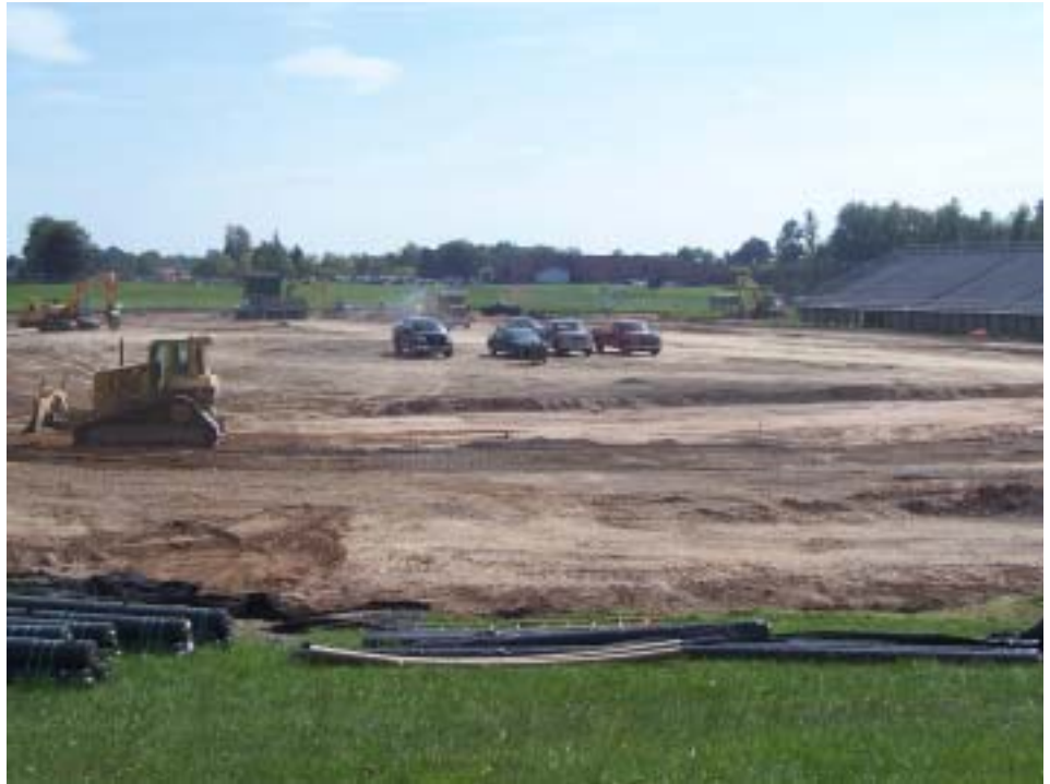
Despite initial delays, work is progressing at the high school on major renovations to the athletic complex. (Senecal photo)
