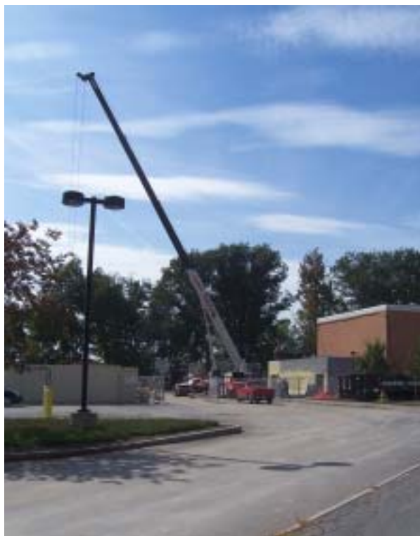
The locker rooms at GRB will be undergoing a much-needed expansion as part of the ongoing construction project. (Senecal photo)
